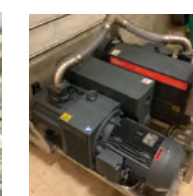
Upgraded vacuum pump outside machine frame
